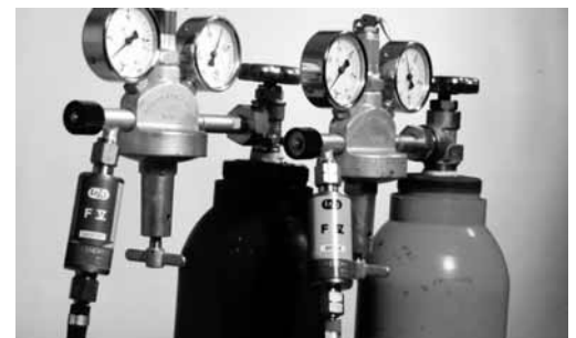
Fig. 6: Gas welding station with pressure reducing valve, non-return valve, flashback arrester.
