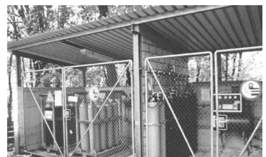
Fig. 7: Explosion protection measures at an outdoor site for gas cylinders and gas cylinder groups for inflammable gases (good natural ventilation, Ex zone 1).
