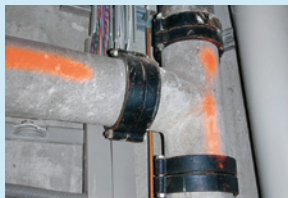
Tubo in fibrocemento
